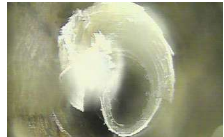
FAILED CIPP LINER
